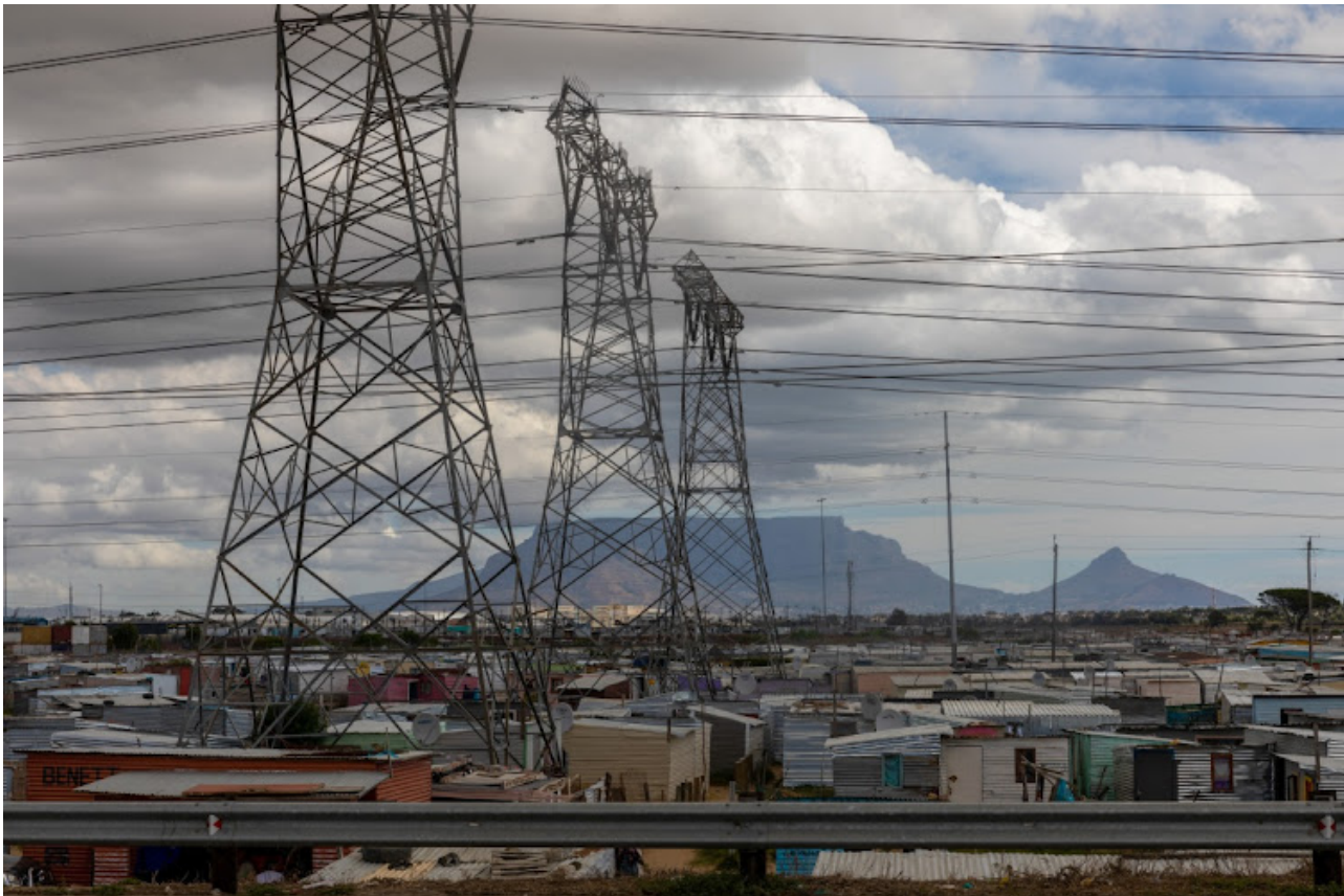
Electricity transmission pylons are shown in the Dunoon informal settlement in Cape Town. Picture: DWAYNE SENIOR/BLOOMBERG
