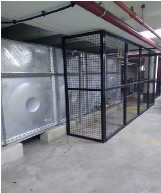
An in-line water back-up system
