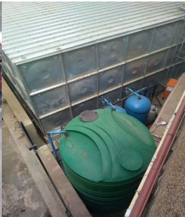
Water storage system
